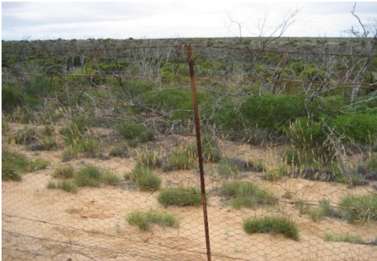
Burnt dropper and brittle wire in a high priority section of Pureba
