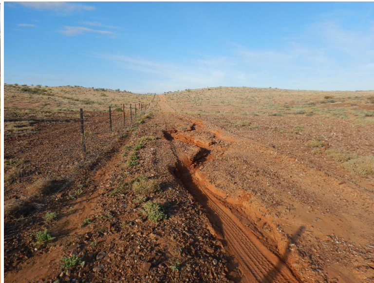
Water damage to track – Mundowdna
