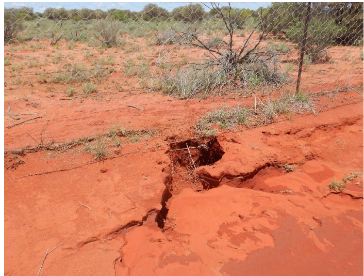
Minor washout next to fence – Mobella (NWP)
