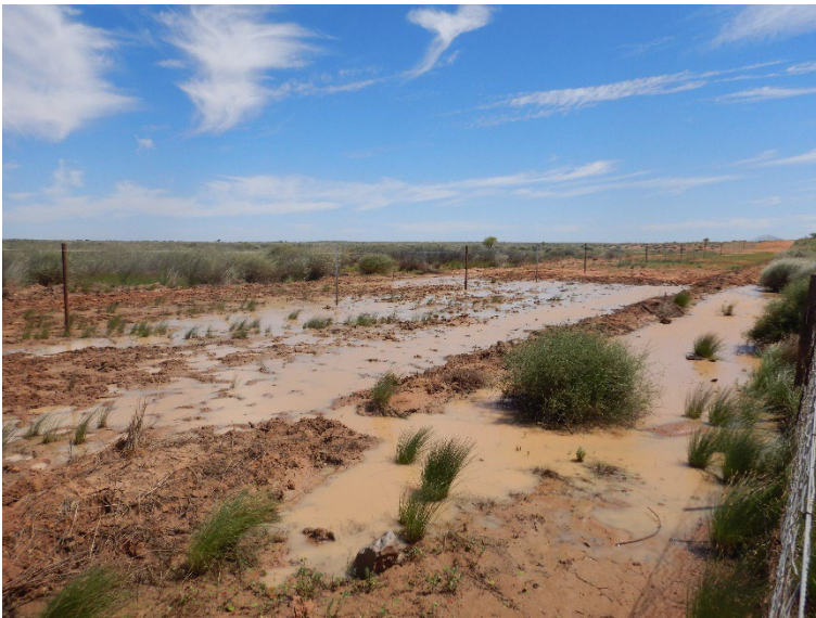
Rainwater over track and Fence – Roxby
