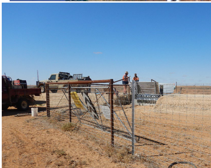
Stock grid installation – Muloorina
