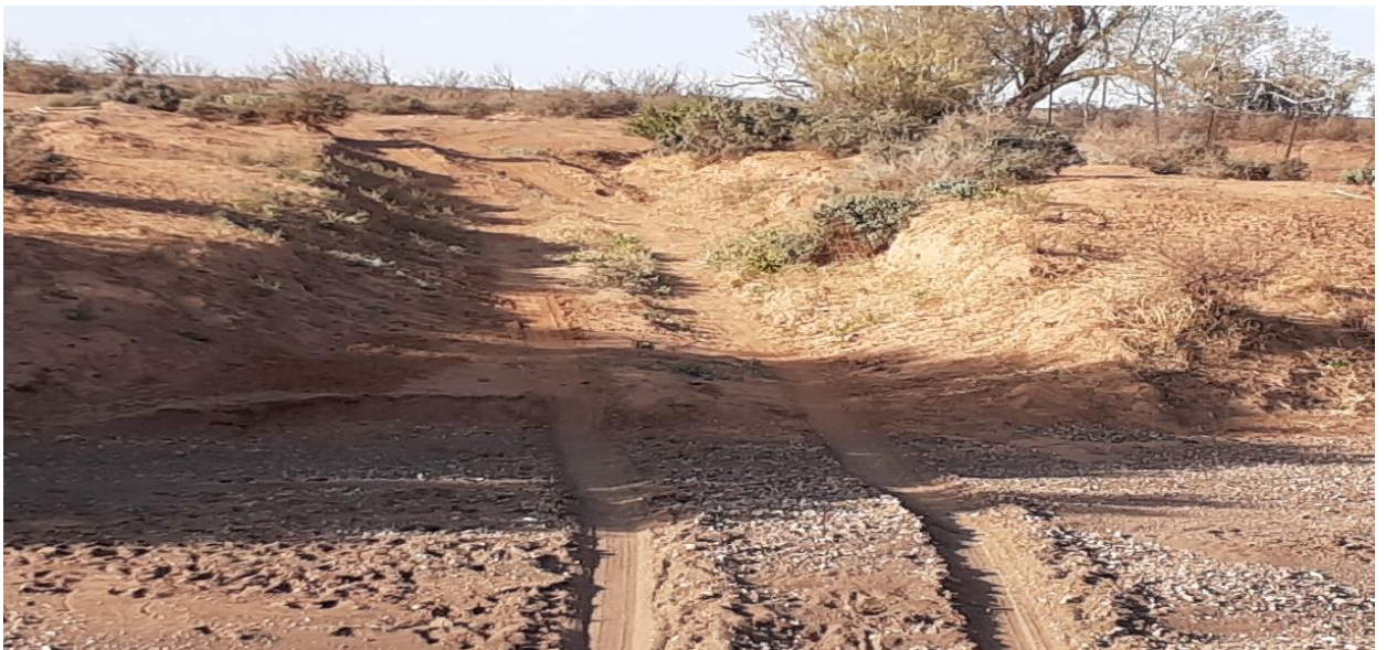
Typical creek crossing – erosion channel developing on entry.
