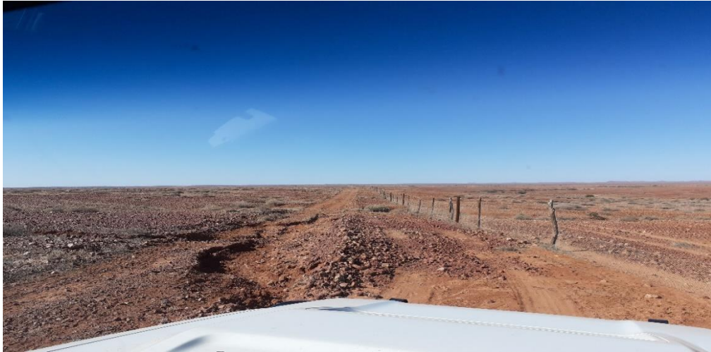
Track erosion requiring work on Millers Creek
