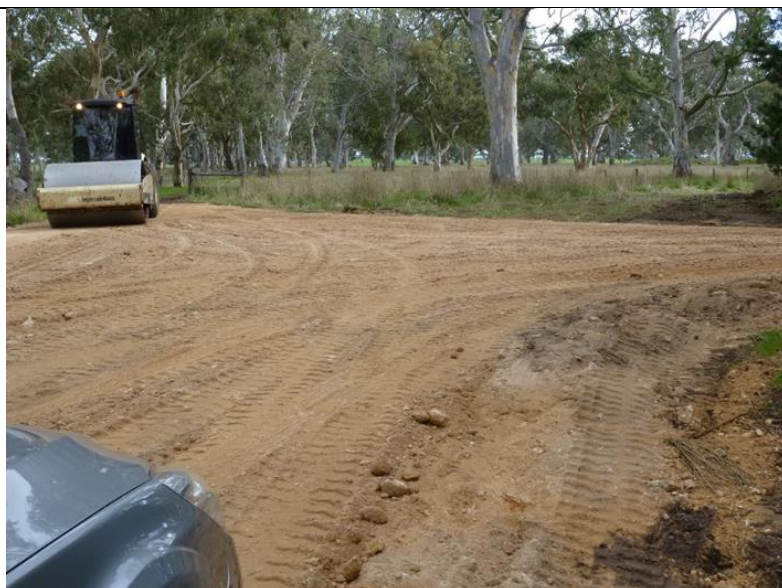
Figure 19: Farm log truck tracks must have allowance for trucks to turn around (Photo by DJ Geddes®)
