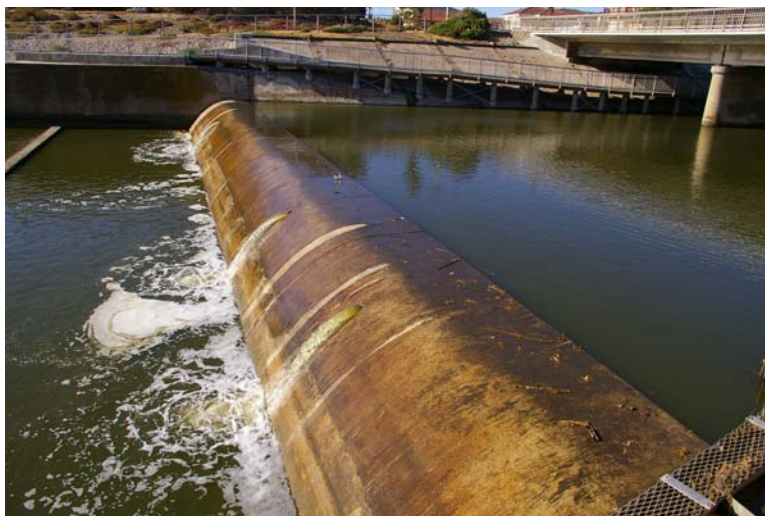
Figure 12. Breakout Creek Weir just above zero-water level, with flow just overtopping the weir crest. Higher abundances of common galaxias and congolli were collected in the exit trap at or below this flow.
